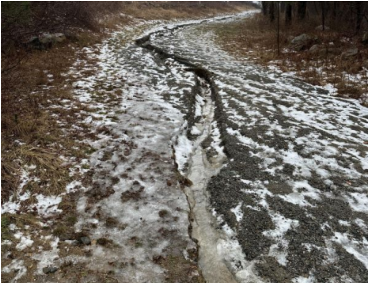
Sagamore Storm Damage
